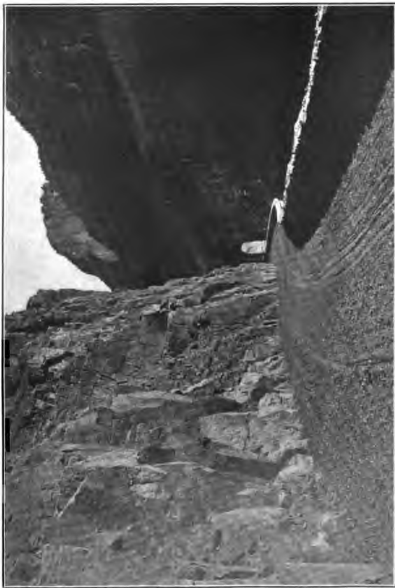
ERECTION OF GOLDEN GATE VIADUCT. TOP VIEW OF COMPLETED WORK FOR ROAD ABOVE VIADUCT.
