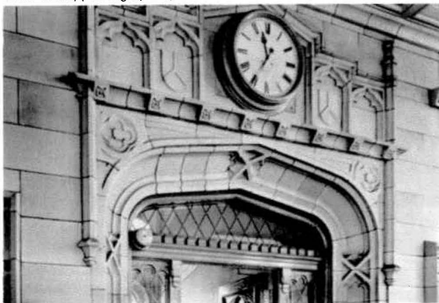
The very fine glazed terra-cotta interior of the Pumping Station dates from the early 1900s. (Bob Thall, photographer)
